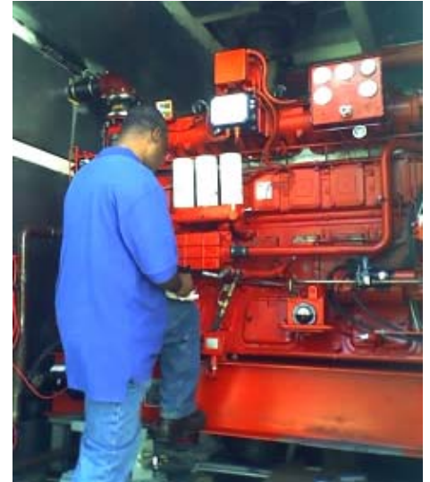
A District mechanical engineer records engine operating data.
